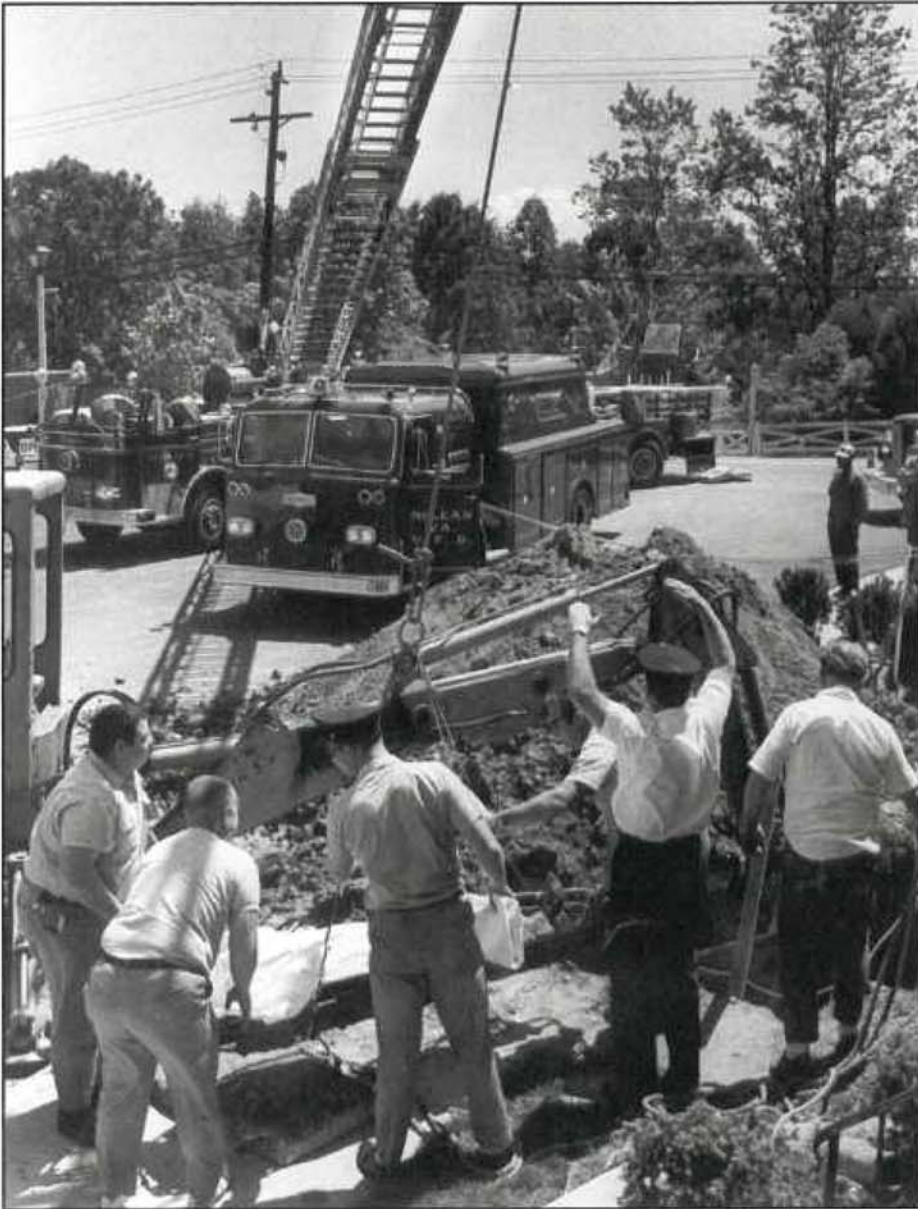
Cave-In at Chain Bridge Road and Halcrest Road. During this May, 1970 incident, a patient was rescued from drowning.
